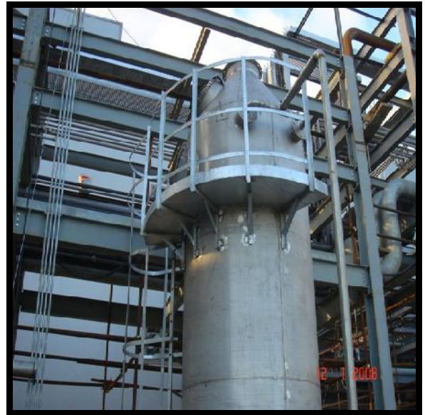
HYO SUNG VOC WET SCRUBBER
