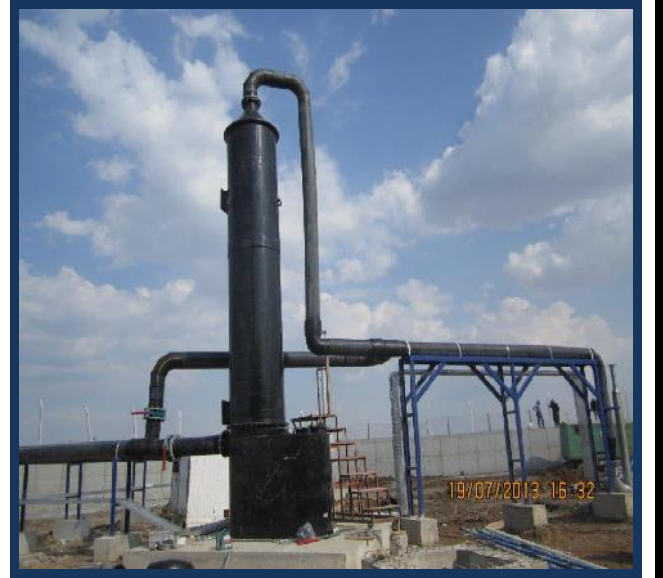
BİYOGAZ WET SCRUBBER
