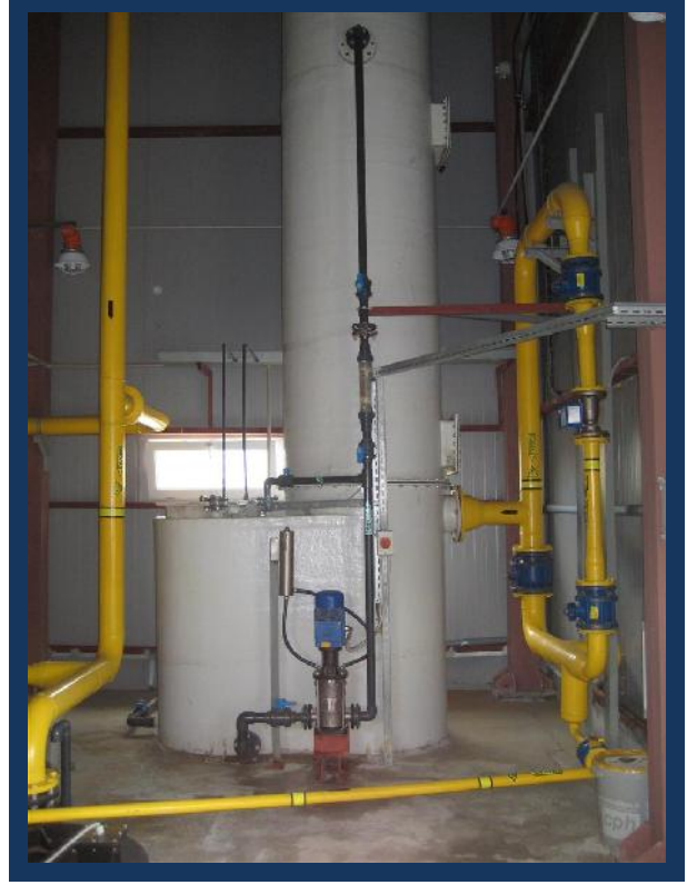
BİYOGAZ WET SCRUBBERİ
