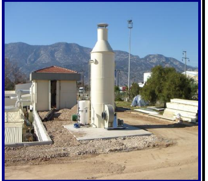
ANTALYA WET SCRUBBER
