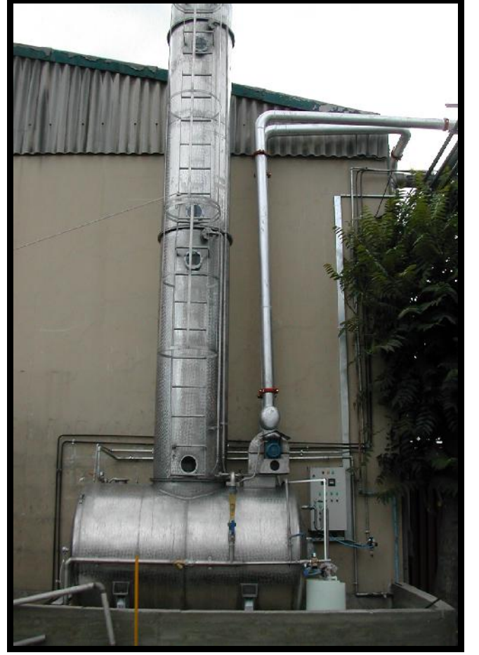
VOC WET SCRUBBER (CLARIANT BOYA)
