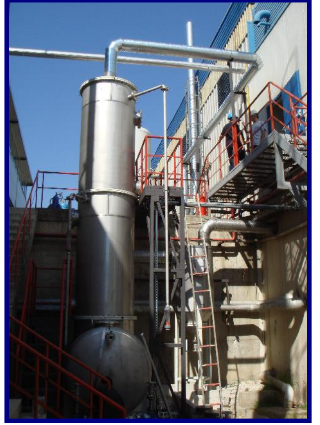
VOC WET SCRUBBER (EGE KİMYA)
