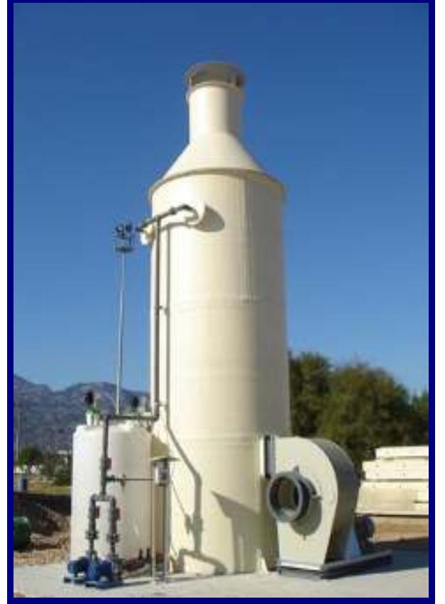
KOKU WET SCRUBBER (ANTALYA OSB)
