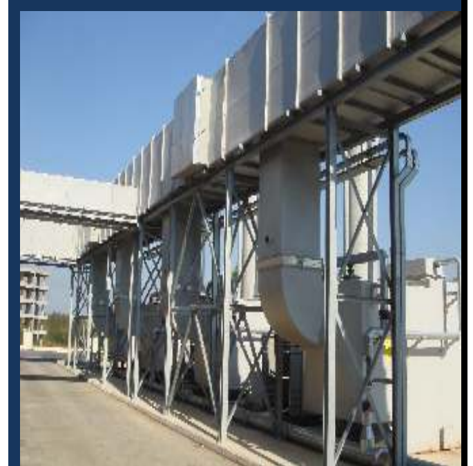
ANTALYA LARA WET SCRUBBER
