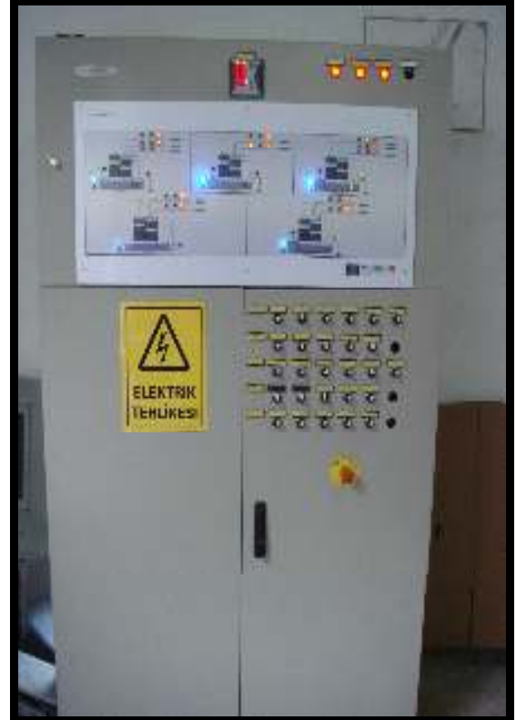
VOC WET SCRUBBER MCC PANOSU
