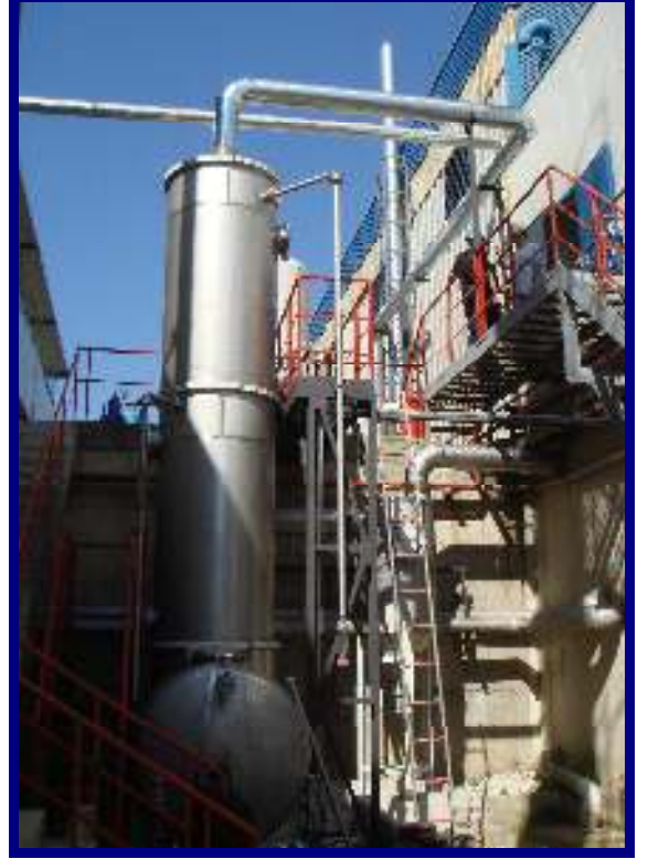
VOC WET SCRUBBER (EGE KİMYA)
